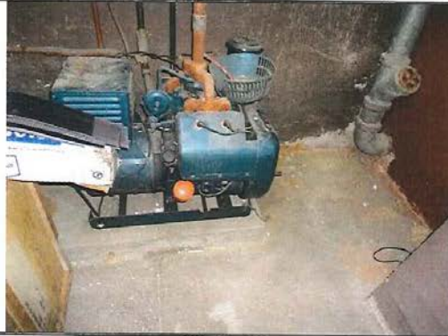
Photo 21 Basement (non-functional natural gas generator)
